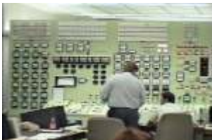
IP2 Control Room
